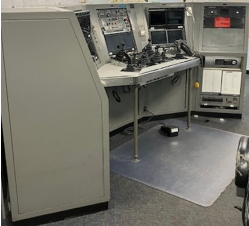
Old Crane Operating Console
