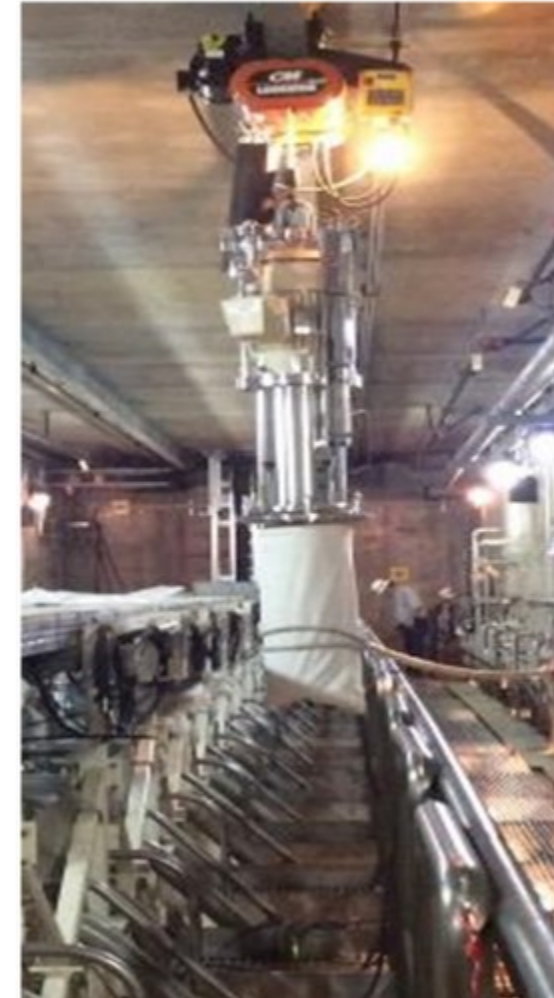
SWPF Centrifugal Contactor
