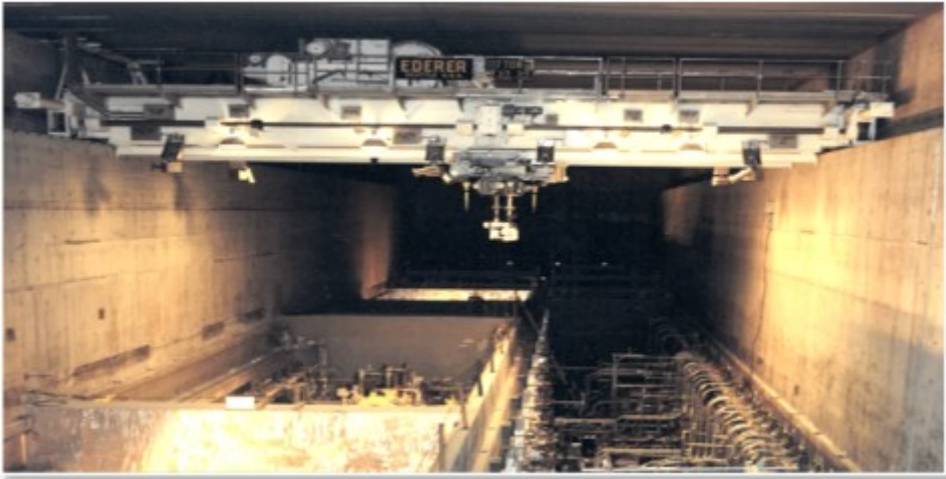
DWPF Main Process Crane (MPC)
